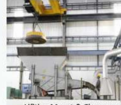
Lifting Magnt & Charger:
